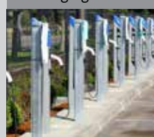
EV Charging Stations
