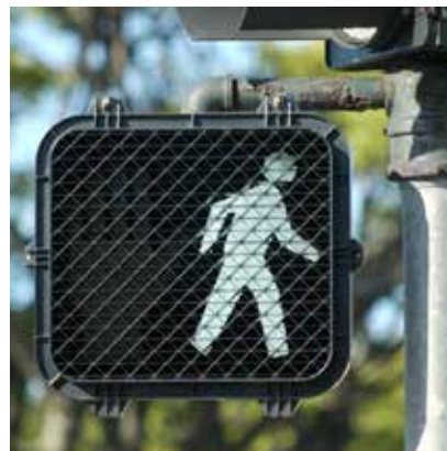
Pedestrian Lead Phase should be considered for Pedestrian safety
